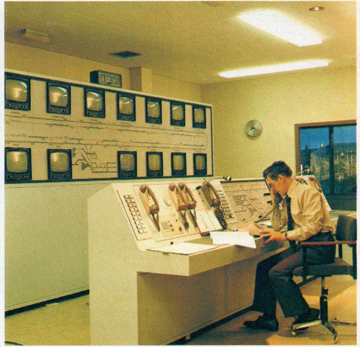
Control room at Broomloan Depot
